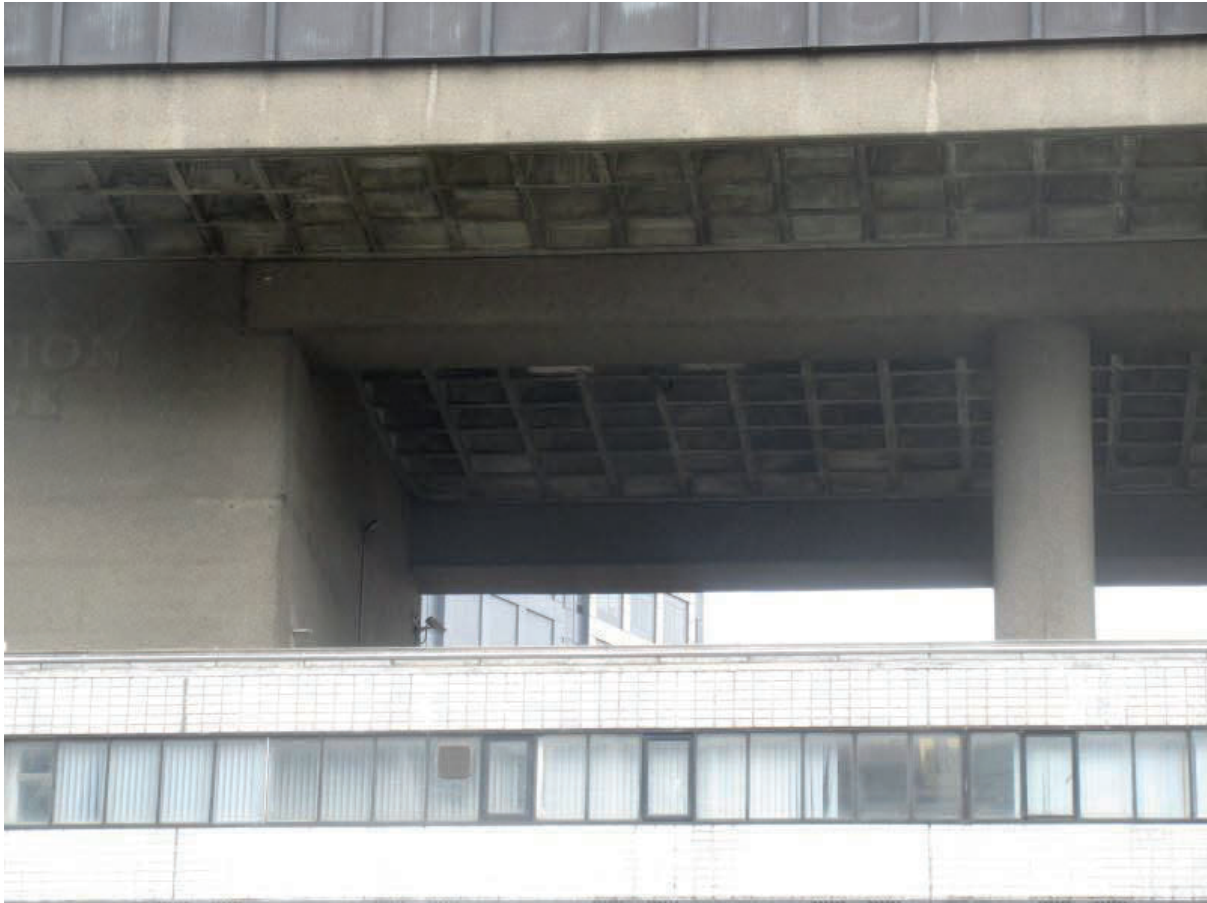
Photo 1 – Soffit of Level 03 – note waffle slab, downstanding part of the beam, column and the south core
