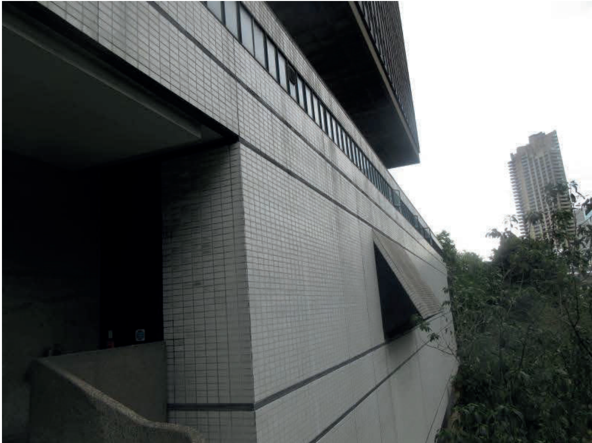
Photo 3 – East elevation of MoL – note extensive use of tiling and their good condition
